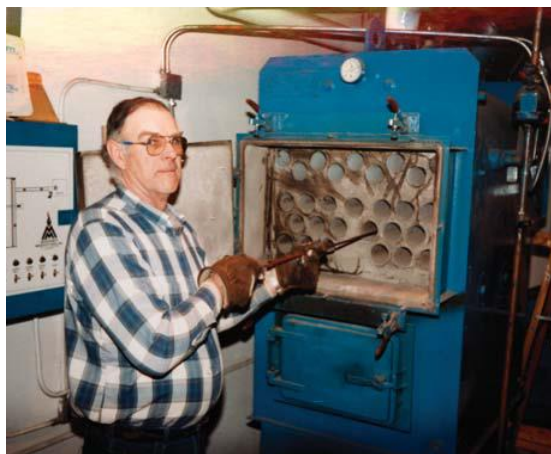
Manual boiler tube cleaning at Calais Elementary School, Calais, Vermont (from the Biomass Energy Resource Center's Wood Chip Heating Systems)
