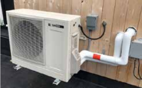
SanCO 2 Eco 2 residential install
