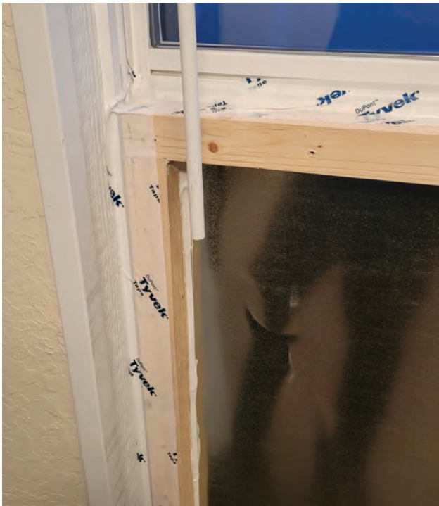
Figure 2-5. Close up of lower window sash replaced with steel sheet metal
