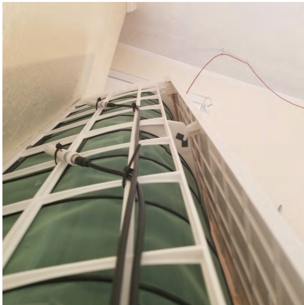
Figure 2-40. System D return/inlet temperature/ RH sensors
