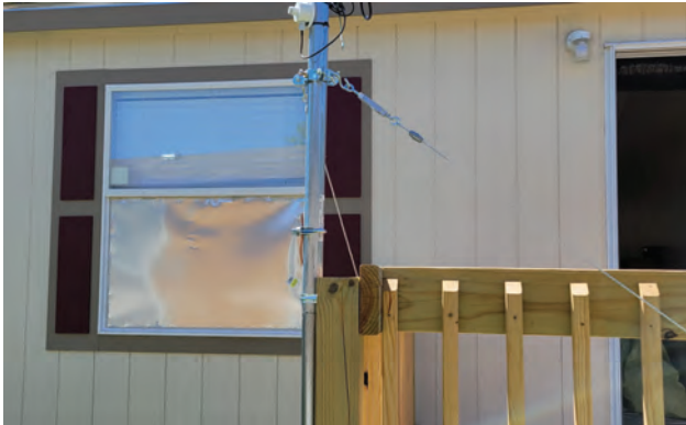
Figure 2-3. House 1 – north-facing window – lower sash replaced with sheet metal
