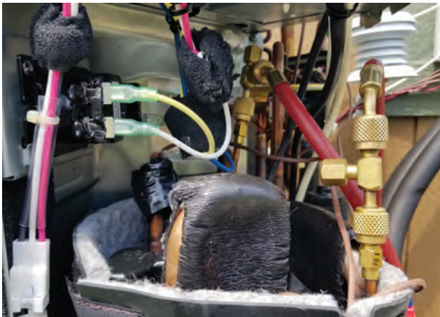
Figure 2-50. Ductless HP, pressure gauge T-tap
