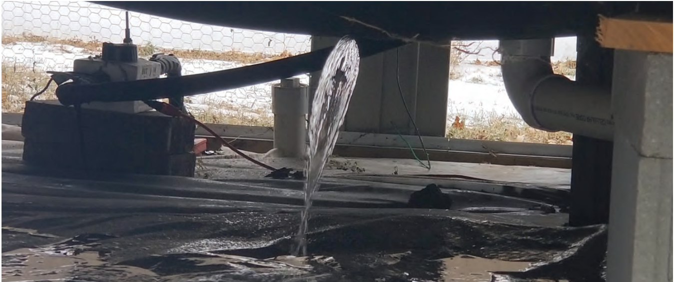
Figure 2-55. House 2 underbelly water leak due to pipe freeze and rupture
