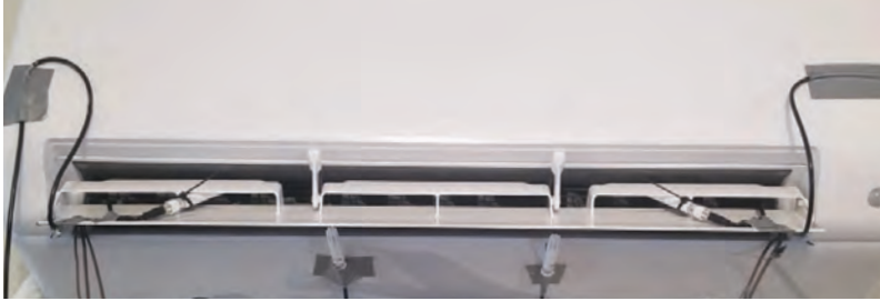
Figure 2-42. Ductless HP supply/outlet air temperature/RH sensors
