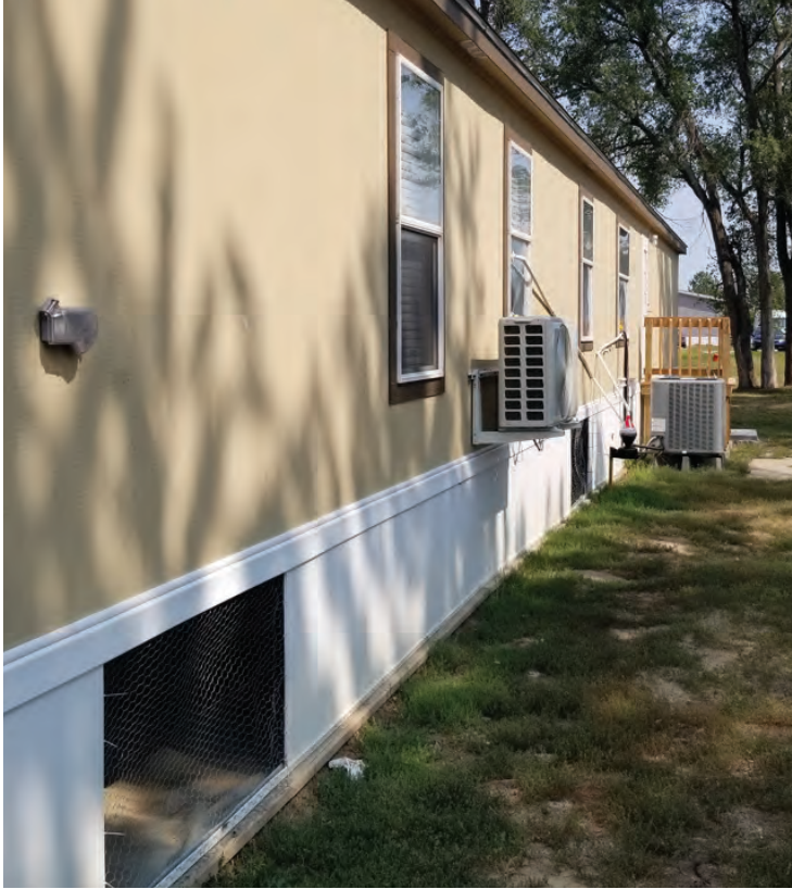
Figure 2-21. House 2 – outdoor units and exposed underbelly
