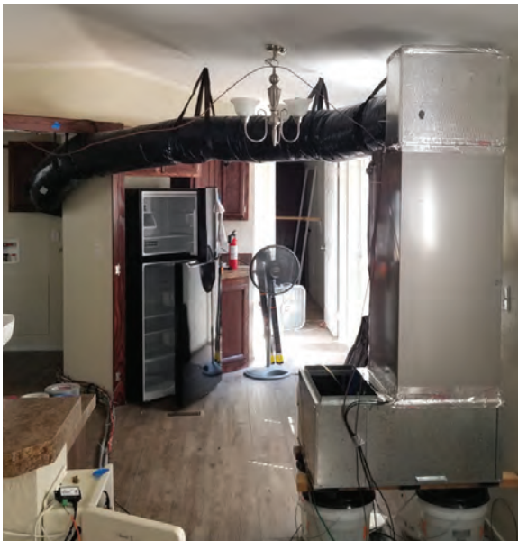
Figure 2-18. System A indoor unit, showing duct
