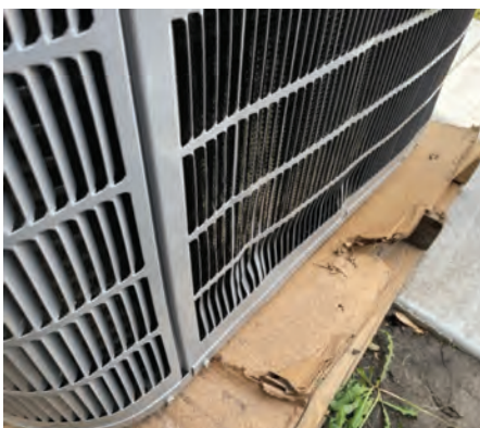
Figure 2-13. System A bent hail guard
