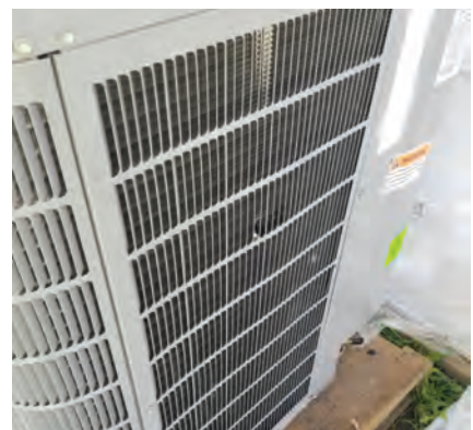
Figure 2-15. System A bent and damaged fins
