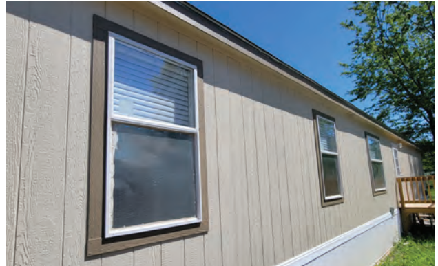
Figure 2-4. House 1 – three south-facing windows – lower sashes replaced with sheet metal
