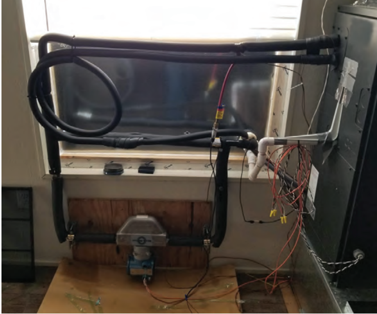
Figure 2-29. System C indoor unit line set and mass flow sensor
