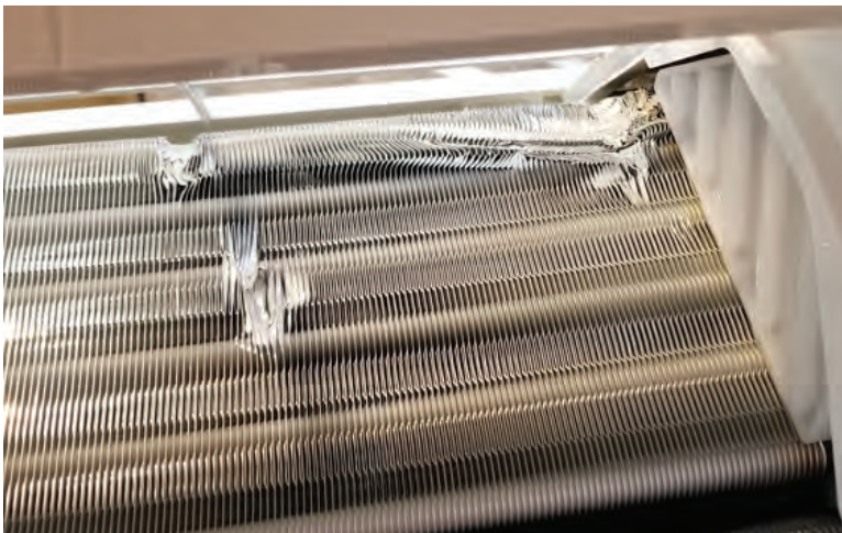
Figure 2-30. System F fin and tube damage
