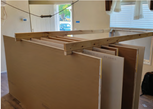
Figure 2-10. Drywall sheets installed in living room area to increase shallow thermal mass
