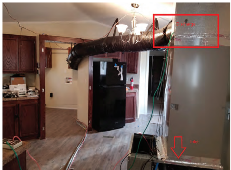
Figure 2-56. Probe location for inlet and discharge, system A
