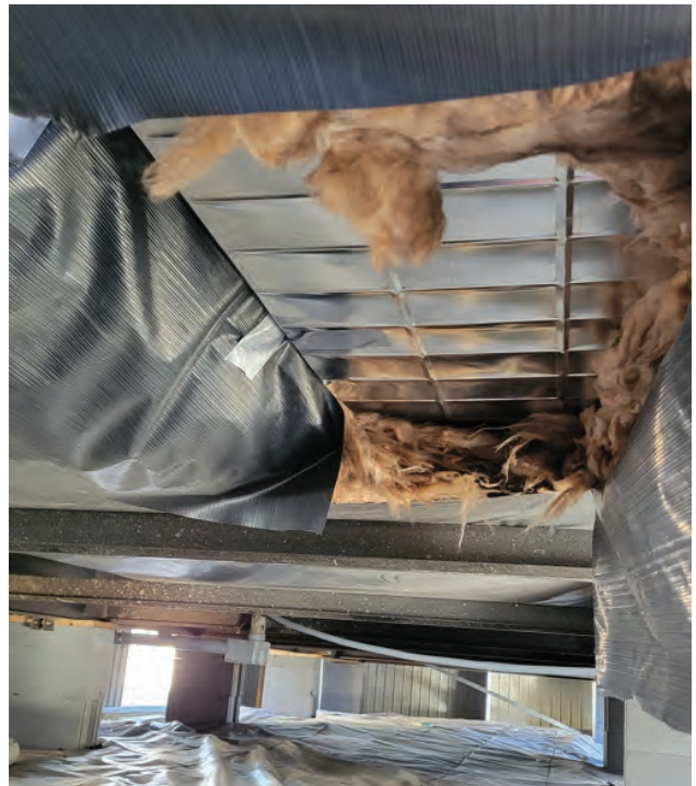
Figure 2-6. House 2 – Section of supply ductwork exposed to increase conductance
