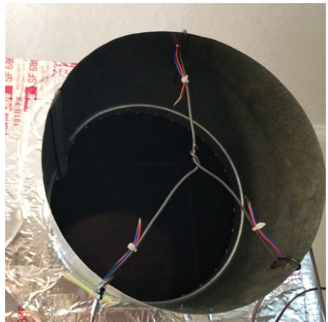
Figure 2-41. System C supply air plenum thermocouple array
