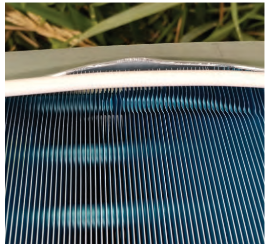
Figure 2-31. System F fin damage
