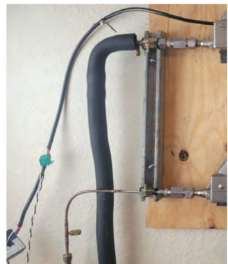
Figure 2-36. Two CTs (one rated 1A and one rated 5A) measuring indoor unit power
