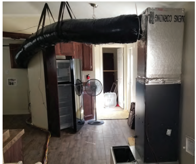
Figure 2-28. System C indoor unit and duct
