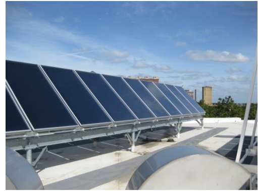
Solar panels at Providence Career and Technical Academy in Providence, RI
