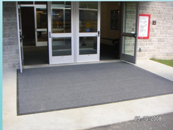
Walk off system at New Hampshire school
