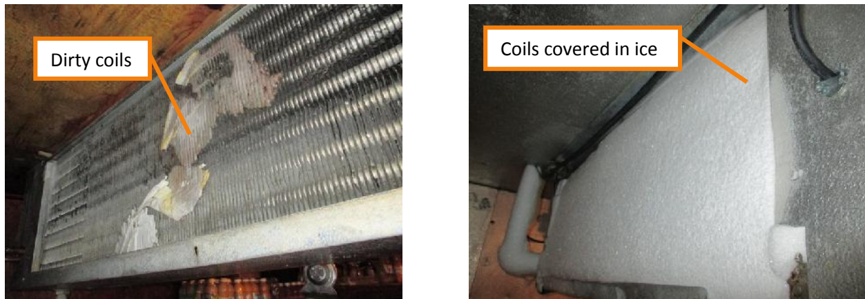
Figure 5. Examples of Poor Evaporator Coil Conditions
