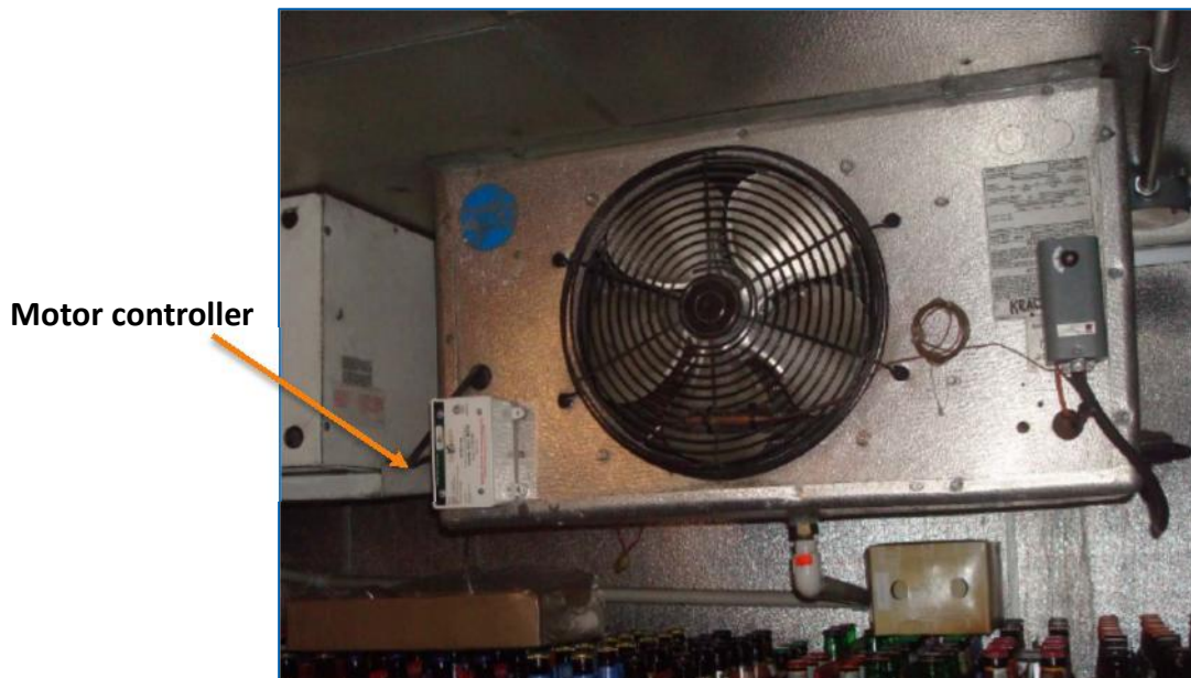
Figure 10. Example of EF Motor Controls in Walk-In Cooler
