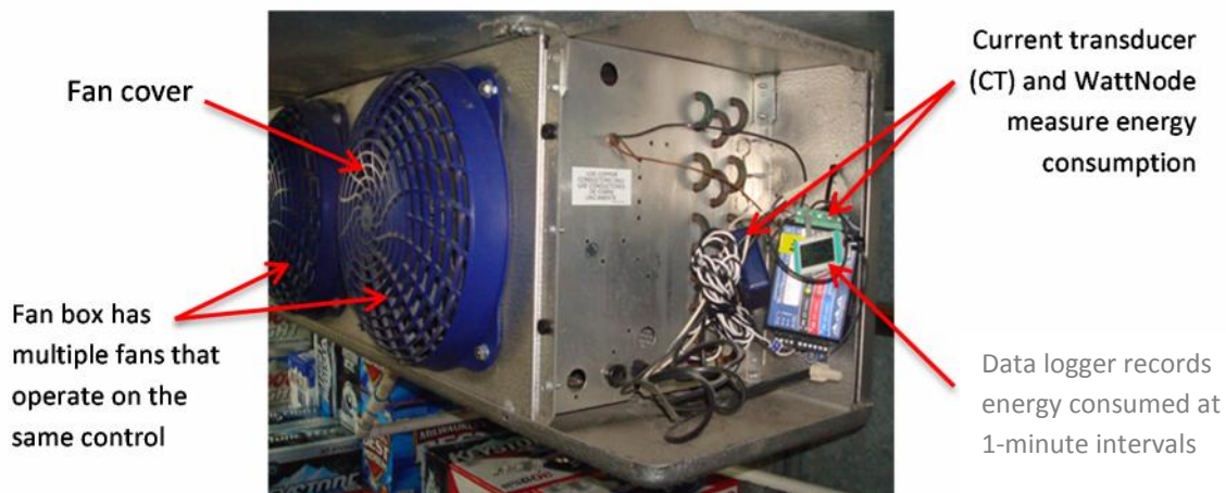
Figure 23. Example of Meter Installation on Evaporator Fans
