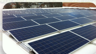
Solar PV system on roof
