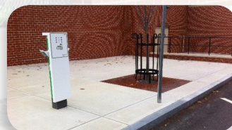
EV charging station
