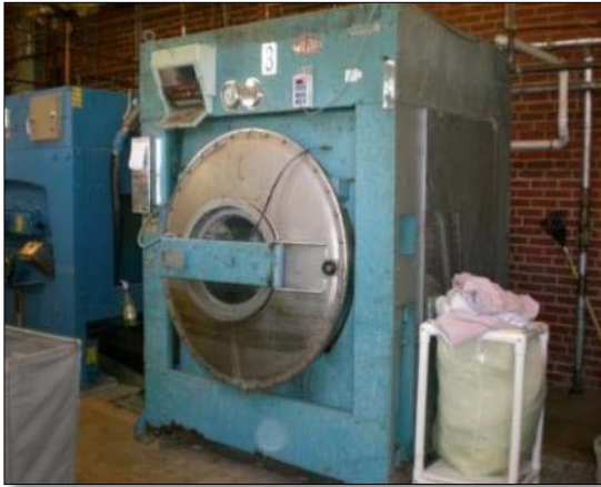
Above: Former Laundry fit at Barron Center, which after retrofit saves the city $104,000 annually.
