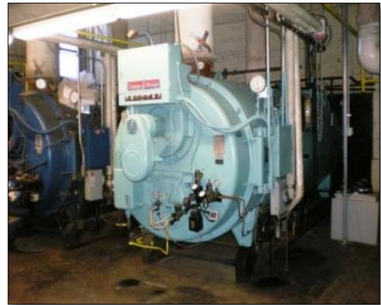
Above: Former oil-fueled boiler at Deering High School, which has been retrofit to instead use natural gas or fuel oil.
